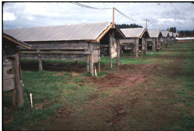
Figure 6. Electrical cables strung from barn to barn to supply power for lights and heat cables.
