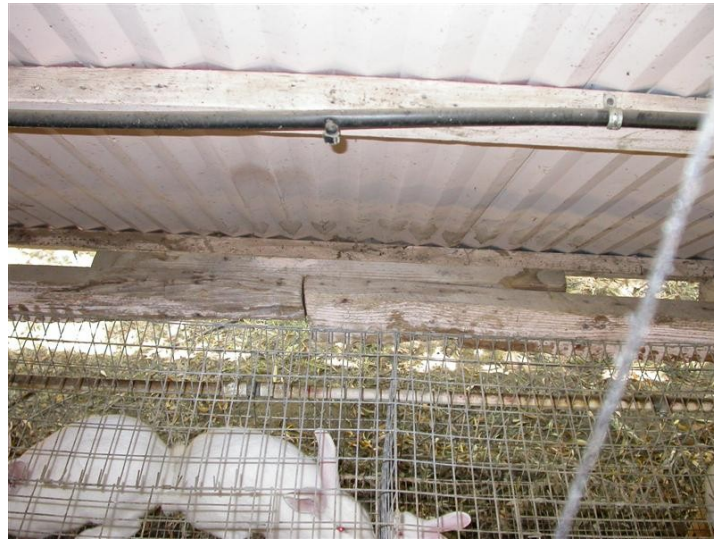
Figure 5. The position of the misters in the A-Frame barn.
